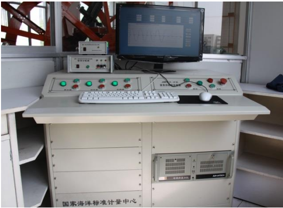
Data acquisition and control system
