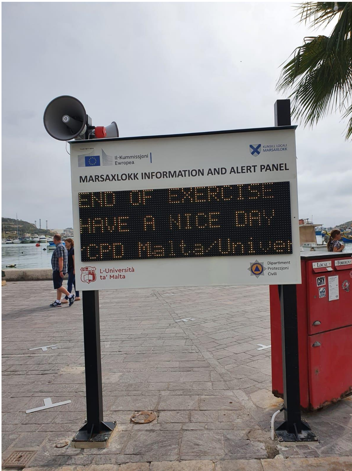
Figure 38: TAD panel showing message of "end of exercise"
