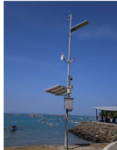
Smart Poles at four locations
