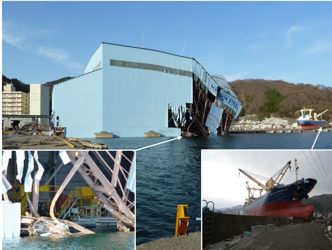
Ship impact damage to steel framed building on piled foundations in Kamaishi
