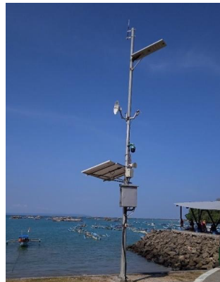
Smart Poles at four locations
