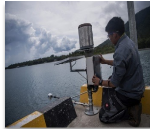
AWS - WATER LEVEL
