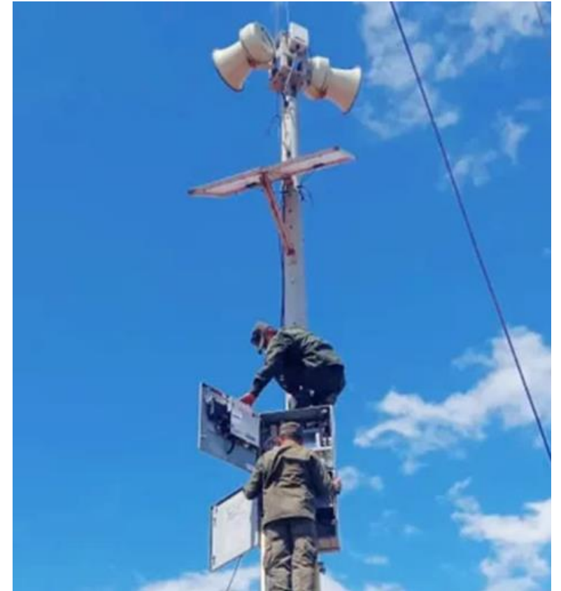
Maintenance of Sirens by Civil Defense of Nicaragua
