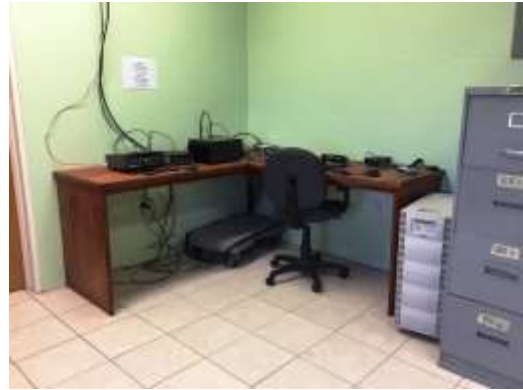
Figure 23. Communication equipment within the Community EOC which supports RESP-3.
