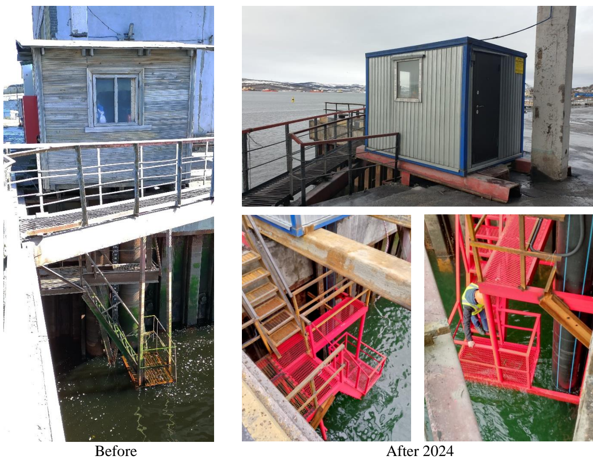
Figure 2. The restored the mareographic pavilion and the stilling well at Murmansk station.
