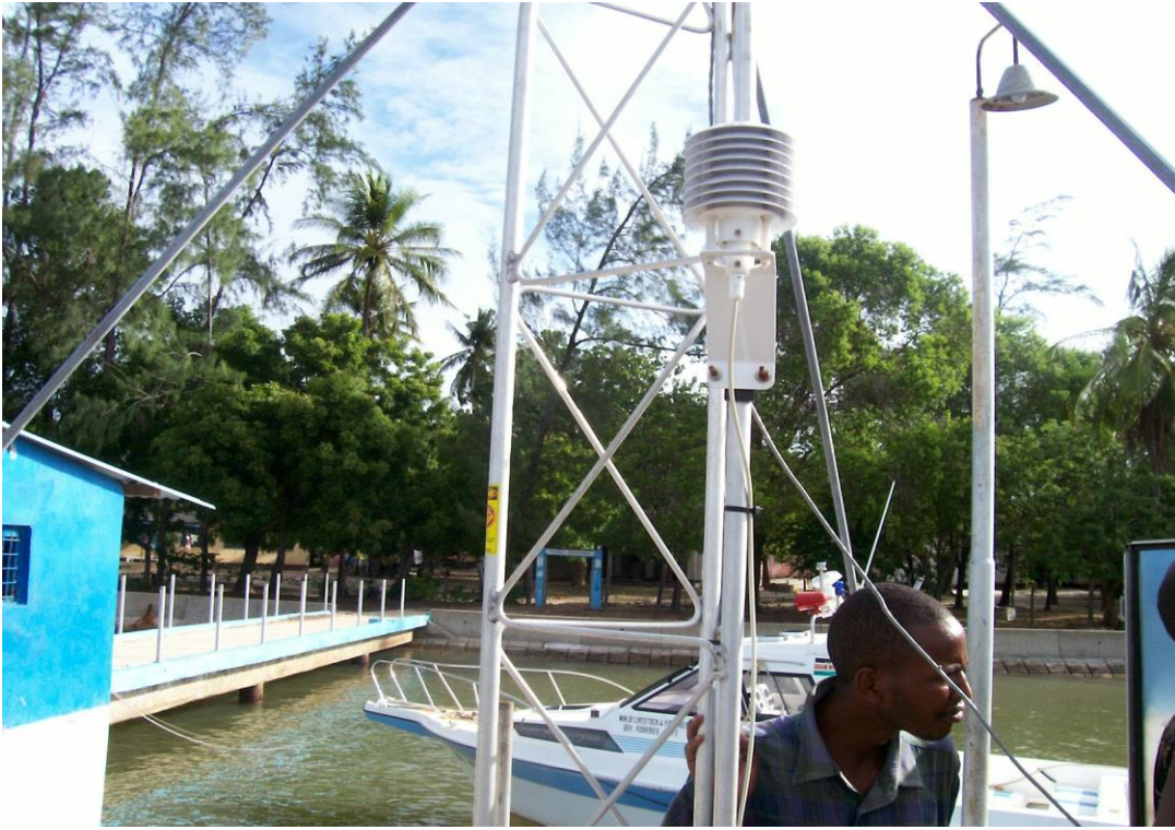
Fig 6a: Lamu Island Automatic Weather Station, at the New Fisheries Jetty.
