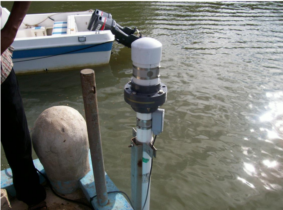
Fig 6b: Stilling Well of tide gauge at New Fisheries Jetty in Lamu Island.
